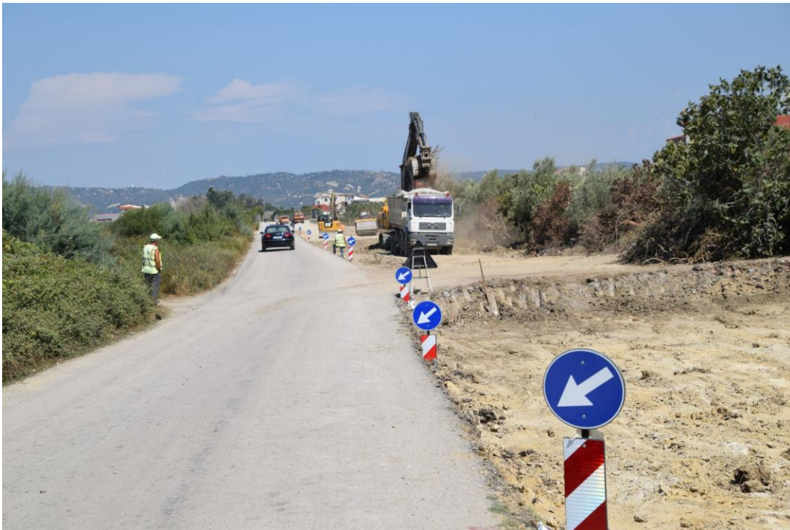
(18) The widening of more than double width of the road which connects the airport with the highway
